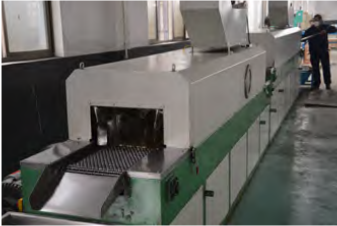
Cleaning + oiling line
